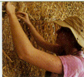
Cover flat portions of bale walls inside and out with standard chicken wire.
