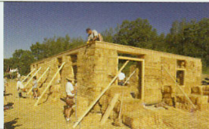
Left and right: Extra bales come in handy for temporary stairs and scaffolding.
